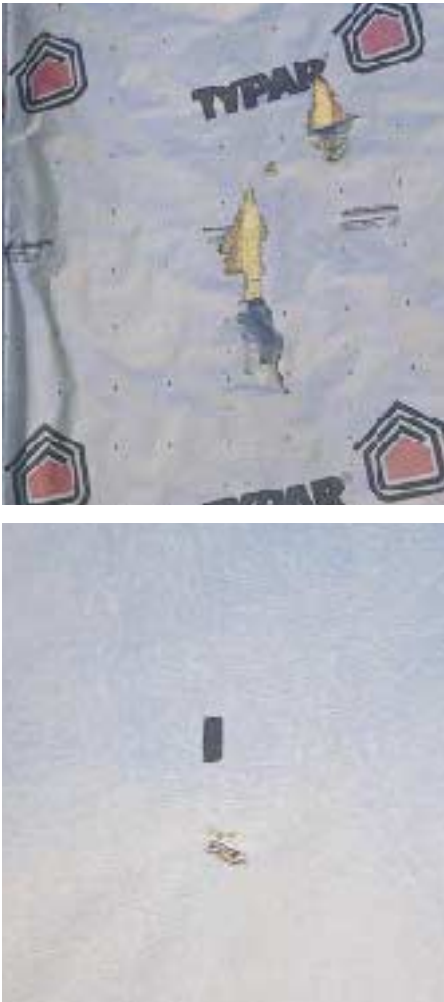
Figure 5. Damage from ladders (top) and tears at staples (above) can undermine an otherwise careful housewrap installation.
