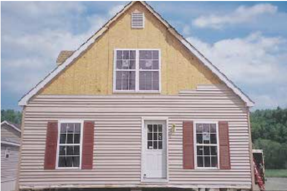
Figure 1. Studies have shown that, on average, houses without a wrap under the siding are more likely to have damp sheathing than houses with felt, kraft paper, or housewrap.
